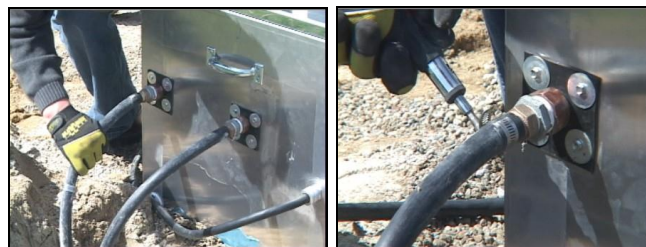
Figure 12. Attach the Loops to the Inlet/Outlets and Secure Them (Your Unit/Connections May Look Different)
