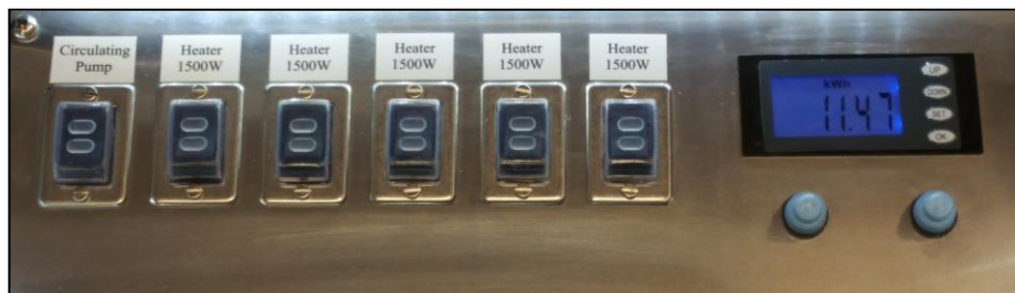
Figure 23. Control Panel with Convenience Meter
