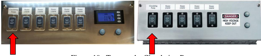
Figure 19. Turn on the Circulation Pump
