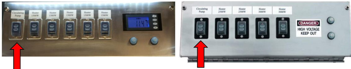
Figure 17. Toggle the Pump
